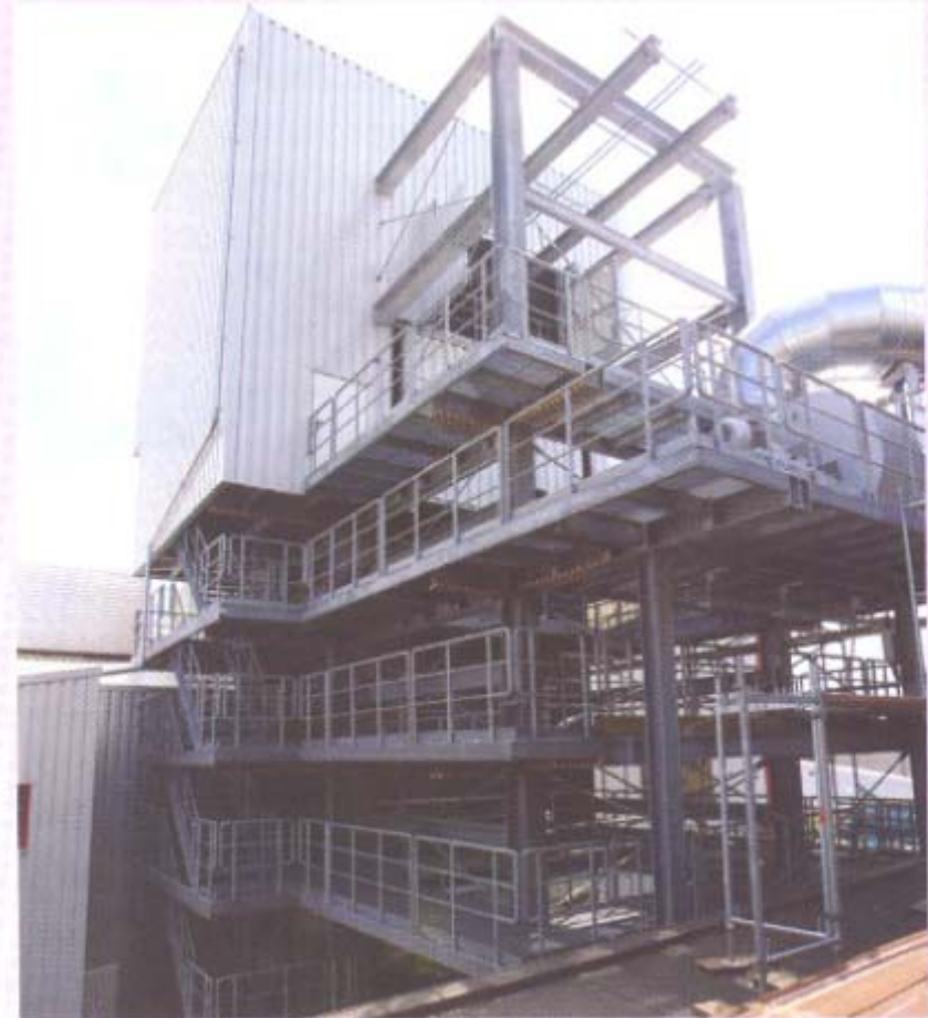
A second SORG batch preheater has been installed at Wiegand-Glas Steinbach.
